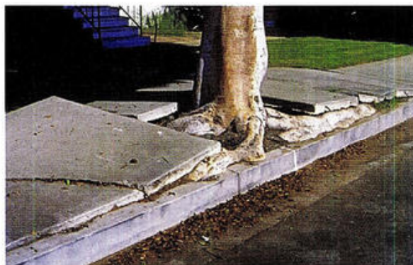
A cracked sidewalk in downtown Newton
