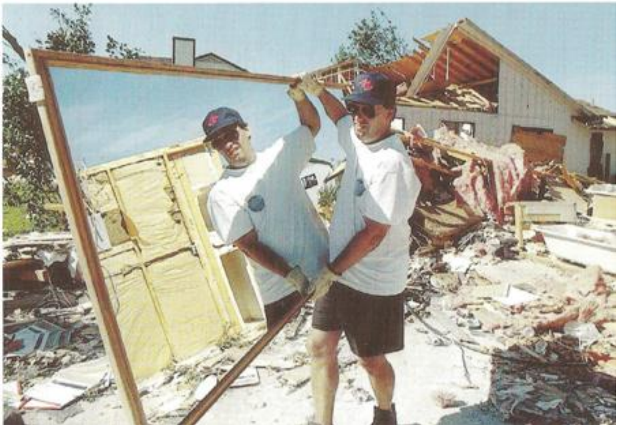
Texas: after a tornado
